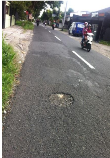
Gambar 5.2 kondisi jalan rating poor
