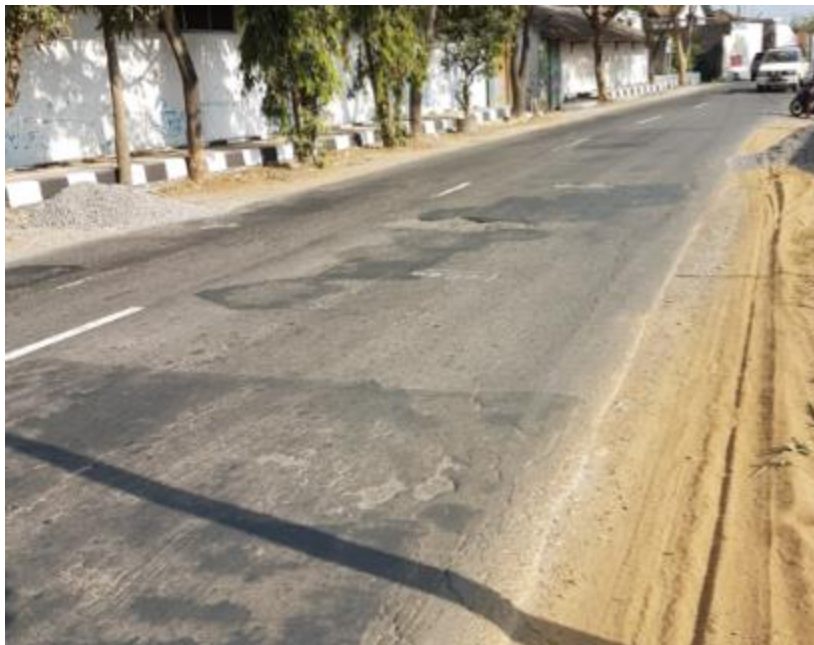
Gambar L-5. 4 Kerusakan Tambalan dan galian ( patching and utility cut )
