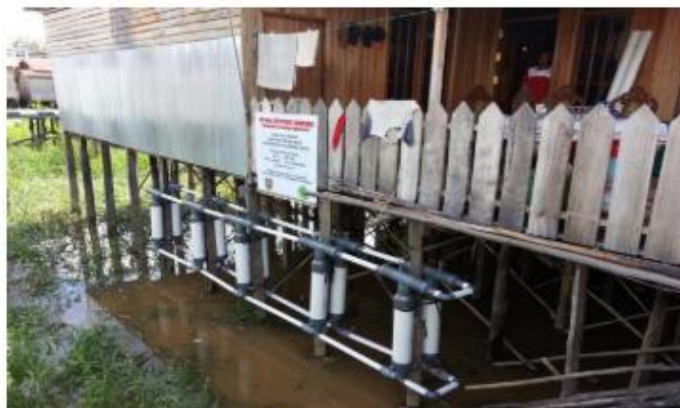
Gambar 2. 5 Repeated Processing Septictank (RPS)
