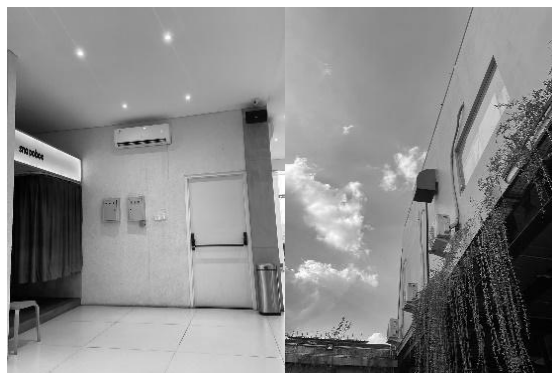
Image 5 Electrical fuses at the storey 3 and exhaust at storey 2 Source : Writer, 2024
