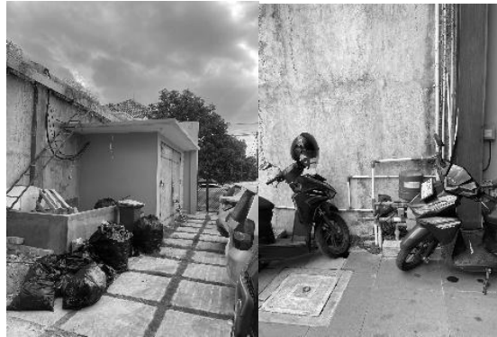
Image 4 Electrical room & water source pump Source : Writer, 2024
