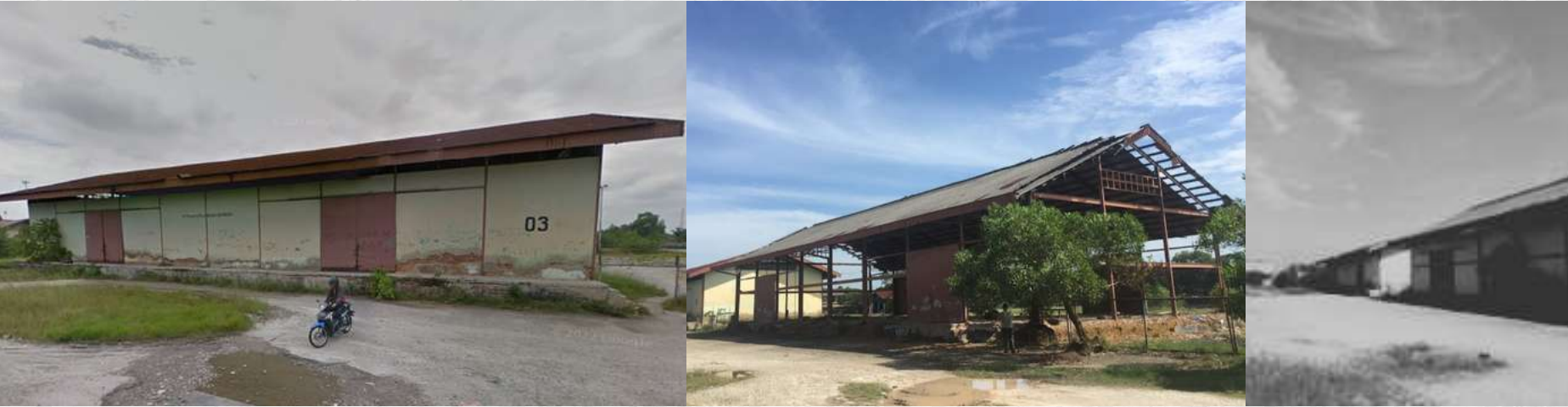
Figure 7,8,9. Condition of the port after being abandoned
