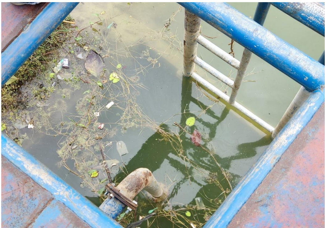
Gambar Pipa Intake
