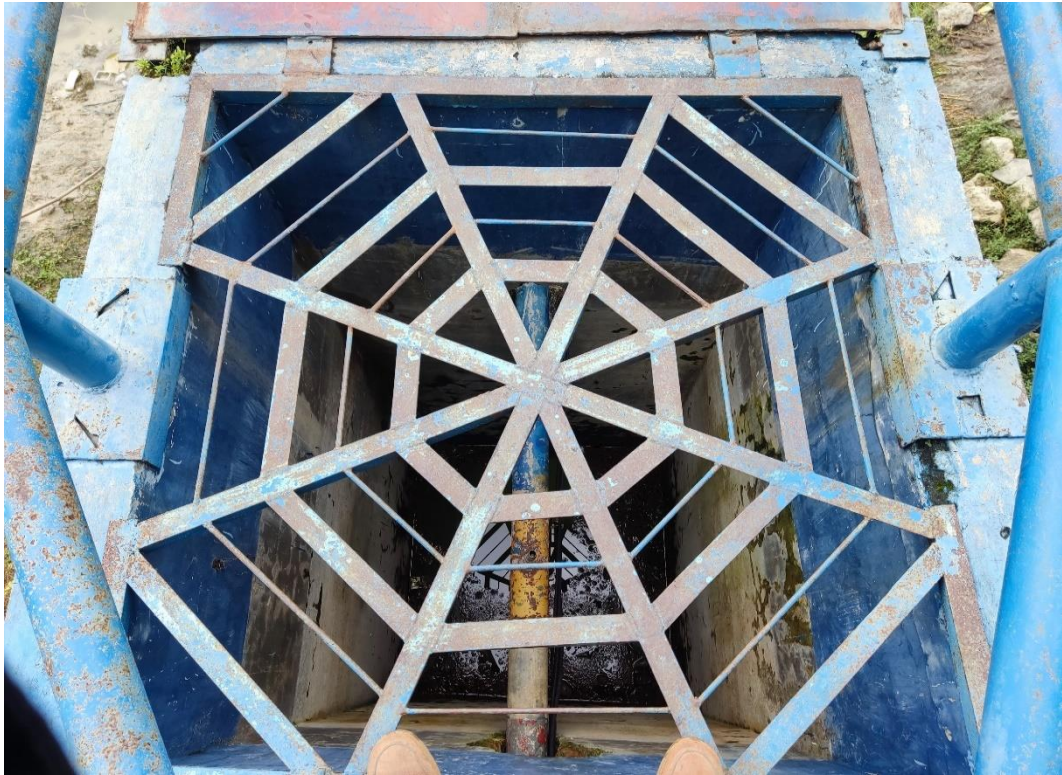
Gambar Pipa Intake
