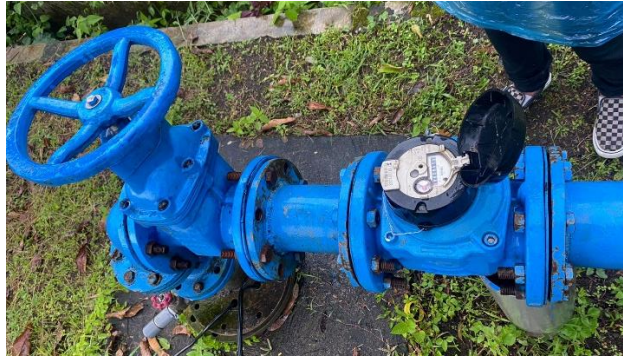
Gambar 4. 4 Sumur 1 PDAM Unit Depok
