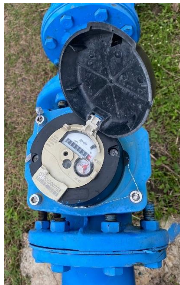
Gambar 4. 6 Water Meter PDAM Unit Depok
