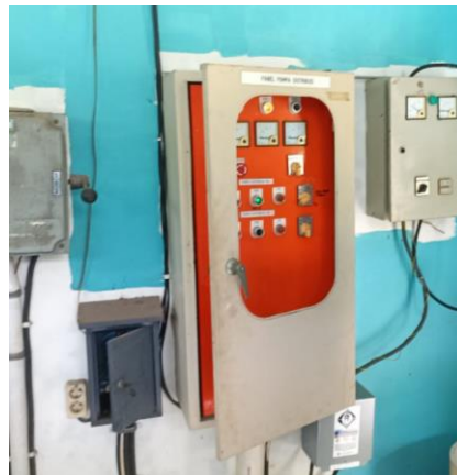
Gambar 4. 11 Panel Listrik PDAM Unit Depok
