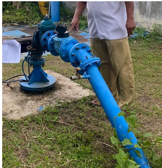
Gambar 4. 5 Sumur 2 PDAM Unit Depok
