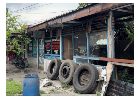
Figure 44: Abandoned building (source: author, 2024)
