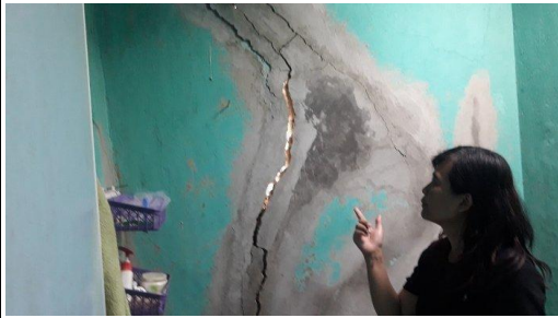
Picture 2. Cracks of one residents home
