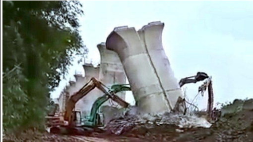
Picture 4. The collapse of the HSR pillar
