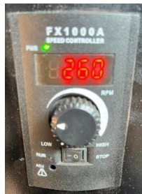
Gambar 4-8 Display speed controller
