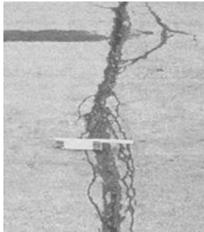
Gambar 3. 7 Contoh Kerusakan Joint reflection cracking
