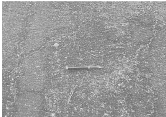
Gambar 3. 11 Contoh Kerusakan Raveling and Weathering
