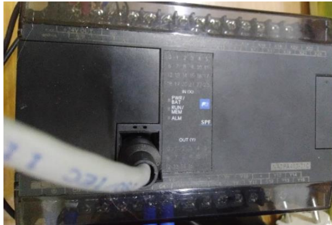
Gambar 3-27 PLC Fuji NA0P40T-31C
