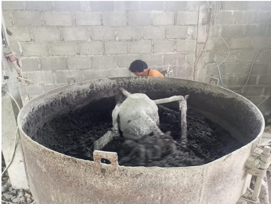
Figure 4.3: The mixer is mixing the material
