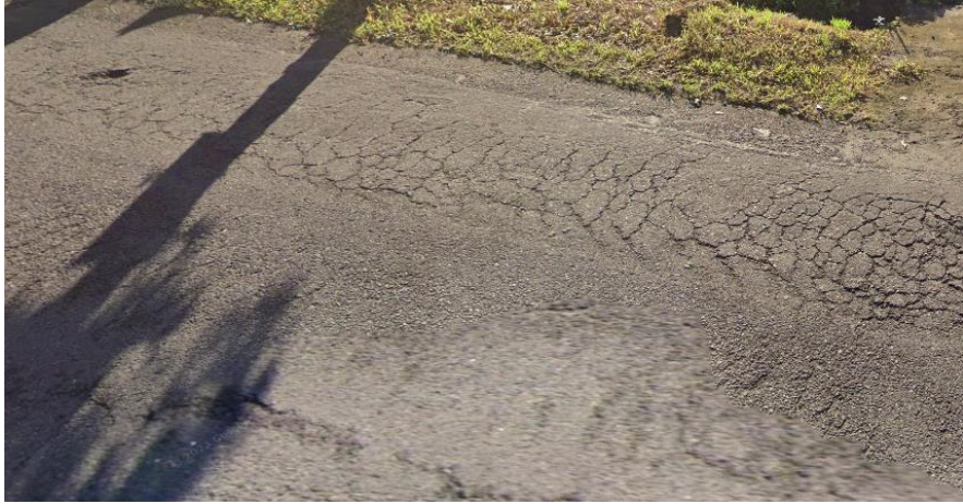
Gambar 7 Kerusakan Block Cracking
