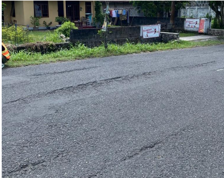
Gambar 3 Kerusakan Longitudinal and Transverse Cracking
