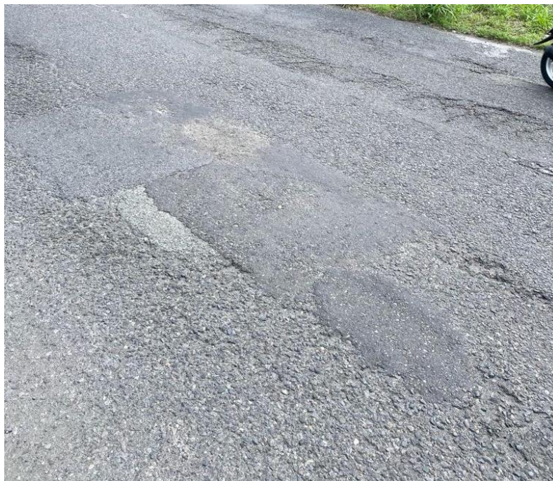
Gambar 4 Kerusakan Patching and Utility Patching
