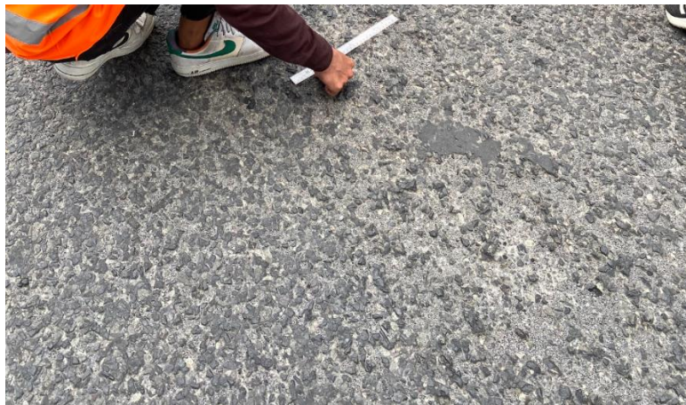
Gambar 2 Kerusakan Polished Aggregate
