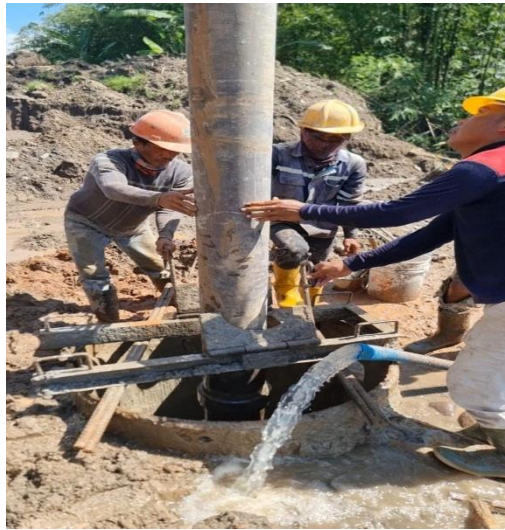
Figure A-1.9 The Process of Installing the Tremie Pipe to the Hole
