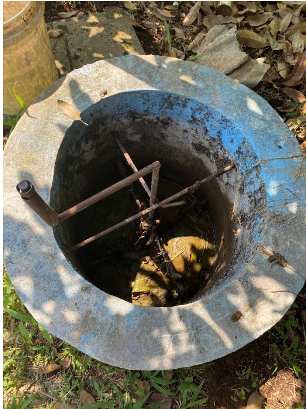
Gambar 3. 4 Mixing Unit Biogas Desa Lau
