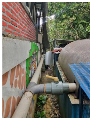
Pipa Influent RBC 1
