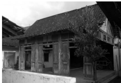
Picture 7 The outer wall of the house before destroyed
