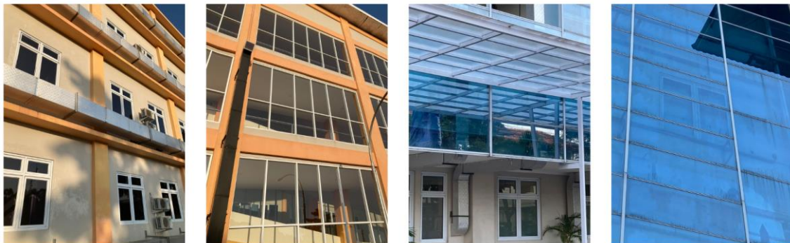
Figure 3 Example of the fenestration types in the building (From left to right, F1, F2, F3, and F4)
