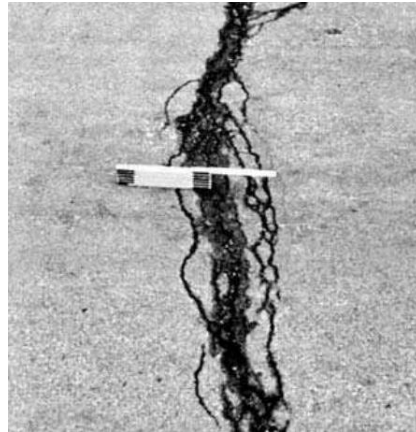
Gambar 3.4 Retak Sambung ( Joint Cracking )
