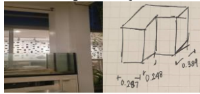
Image 16 and 17 Reinforced concrete Column, L-shaped in Senja Coffee and Memories
