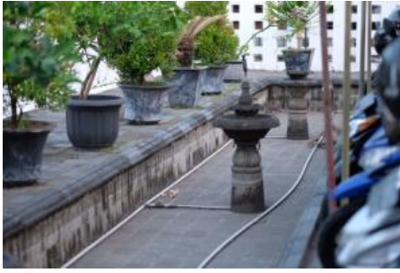
Figure 15. Gutter in Kauman Great Mosque
