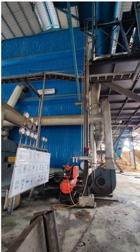
Gambar 4. 15 Mesin Boiler Tampak Samping
