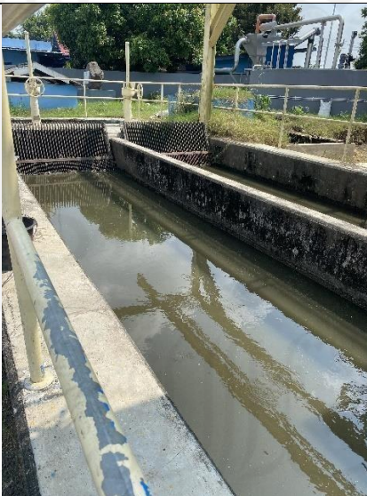
Inlet grease trap
