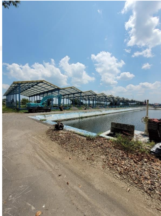
Gambar 4.22 Sludge Drying Bed
