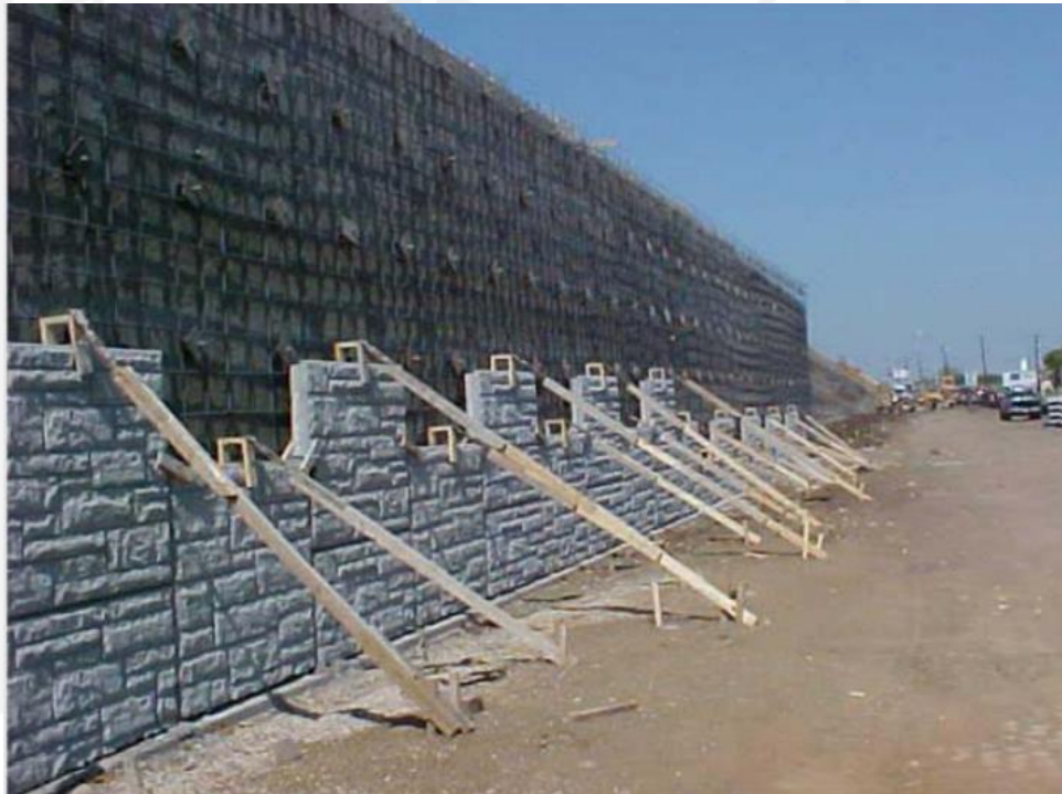
Gambar 3.21 Tampilan Muka Permanen ( Permanent Wall Facing ) (Sumber: "Soil Nail Walls Reference Manual", Report FHWA-NHI-14-007)
