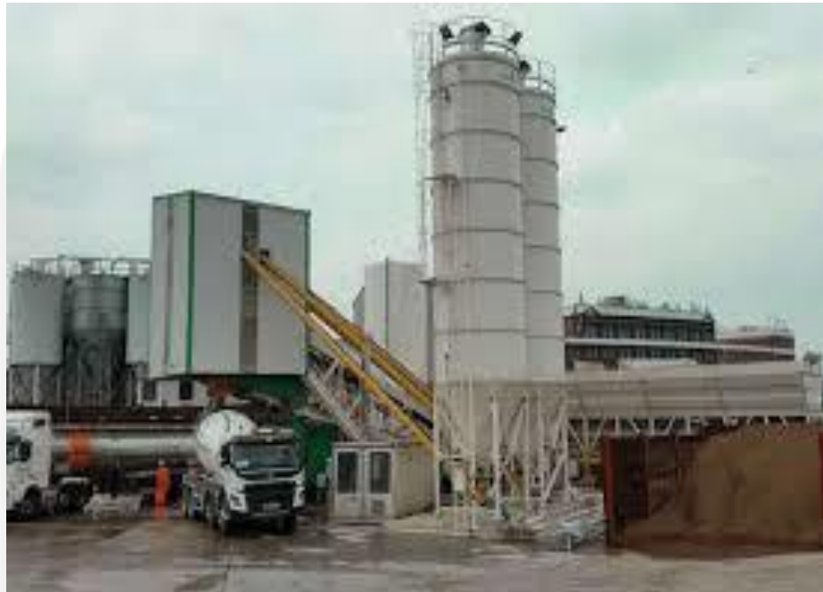
Gambar 3.2 Batching Plant (Sumber: www.readymix.co.id )
