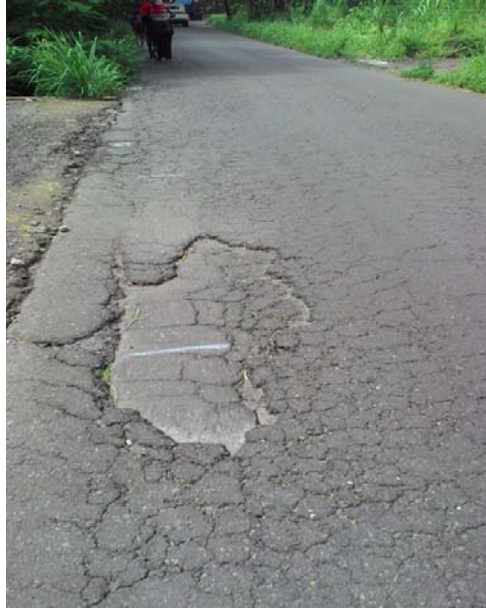
Gambar 5.3 kondisi jalan rating poor
