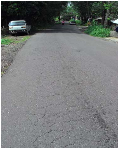
Gambar 5.2 kondisi jalan rating fair
