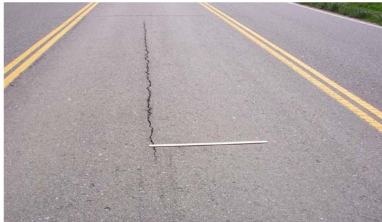
Gambar 3.1 Retak Halus ( Hair crack )
