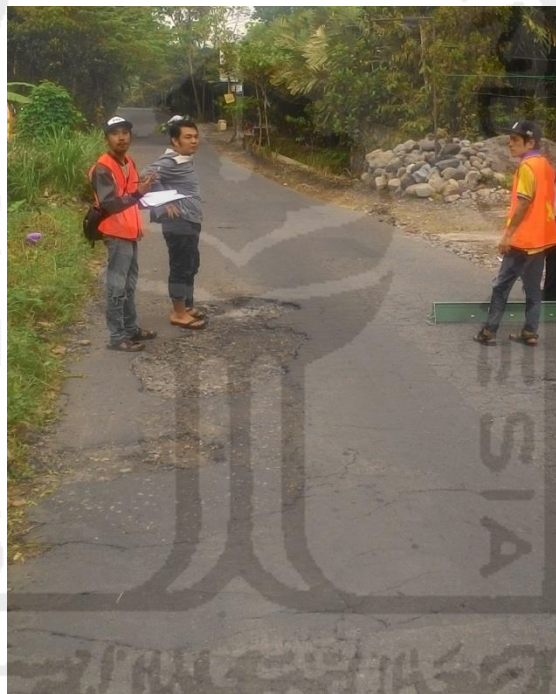
Gambar 5.4 Kondisi Jalan Very Poor (Sumber : Hasil pengamatan, 2016)
