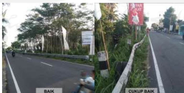
Gambar 5.23 Penilaian Kondisi Guard Rail
