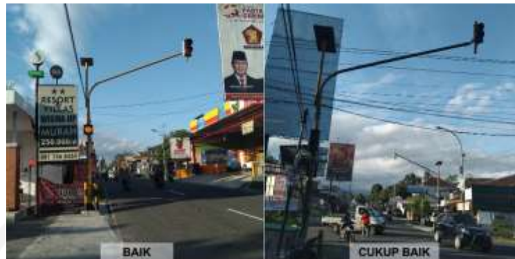
Gambar 5.24 Penilaian Kondisi Warning Light
