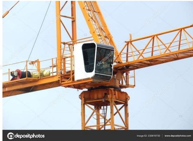
Gambar 3.5 Cabin Tower Crane
