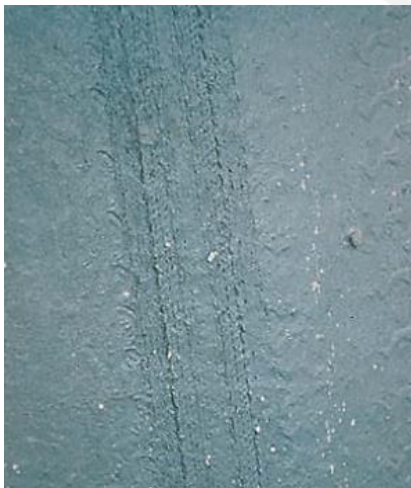
Gambar 3.12 Kegemukan ( Bleeding ) Sumber: Federal Highway Administration (2014)
