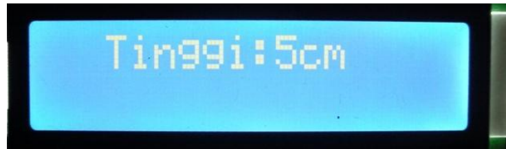
Gambar 4.4 Tampilan Proses Monitoring dan Pengendalian Sistem Drainase
