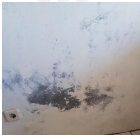
Gambar 5.10 Cat Dinding Interior Terkelupas
