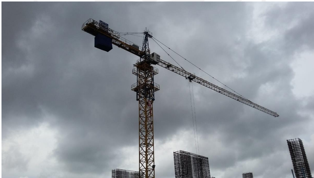
Gambar 7. 1 Tower crane eksisting
