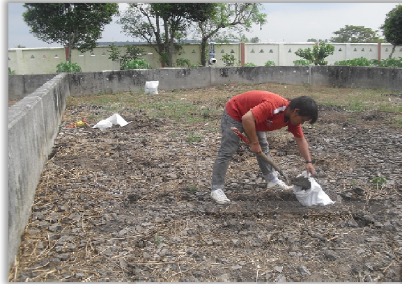
Gambar III.2 SDB ( Sludge Drying Bed ) IPAL Domestik Sewon, Bantul
