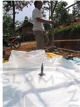
Gambar 2.6. Gas Outlet Terpasang
