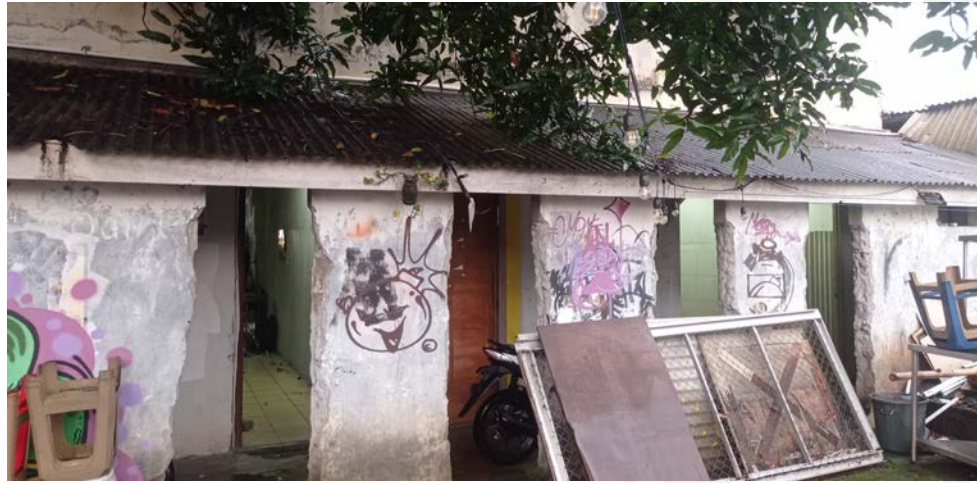
Figure 2.12 Existing condition of Toilet Source : Author
