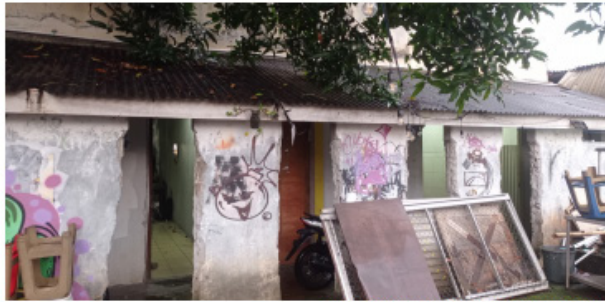
Figure 2.12 Existing condition of Toilet Source : Author
