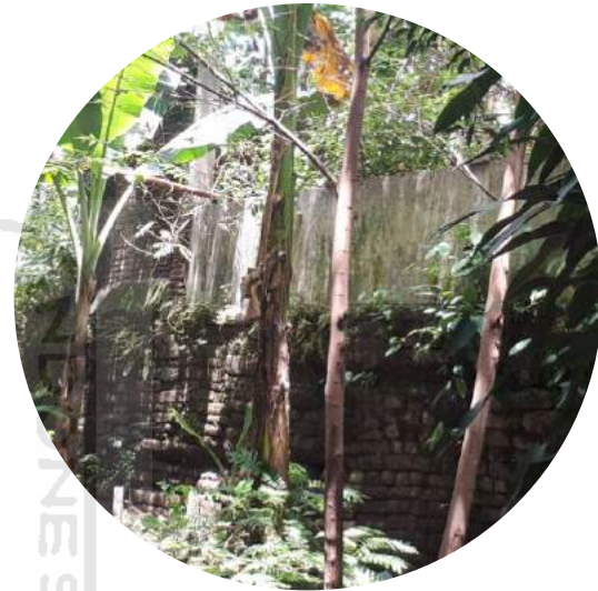
Figure 43. Damaged part of Benteng Cepuri on the north Source: Writer's Document, 2021
