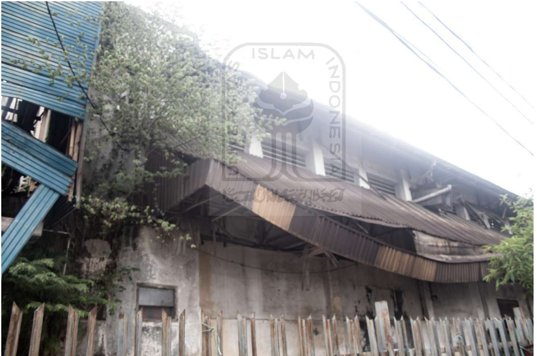
Figure 21: Deformities at the side of the building where the zincalume start to fall apart
