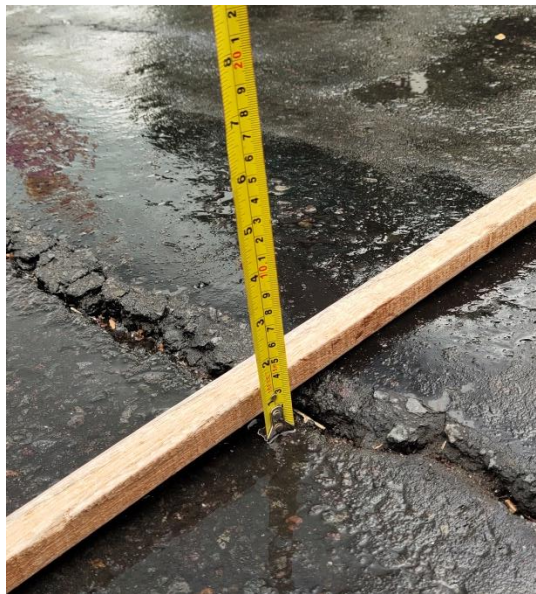
Gambar 5.53 Perbedaan Tinggi Expansion Joint 1 Jembatan Bogem C
