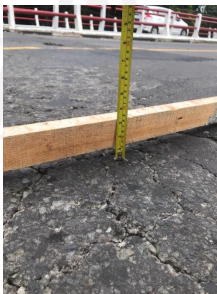
Gambar 5.34 Perbedaan Tinggi Expansion Joint 1 Jembatan Bogem B
