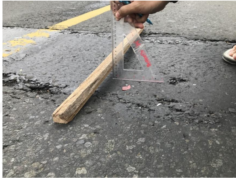
Gambar 5.36 Perbedaan Tinggi Expansion Joint 3 Jembatan Bogem B
