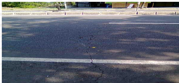
Gambar 3.14 Retak Melintang ( Transversal Cracking )
