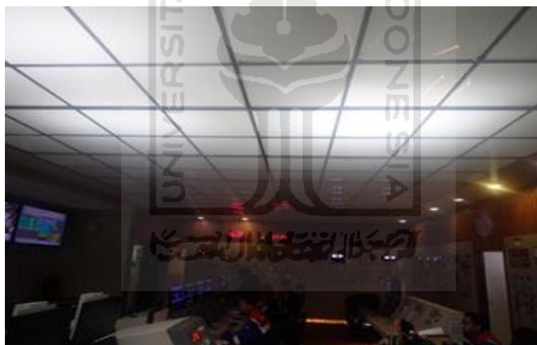
Gambar 4. 1 Control Room Power Plant
