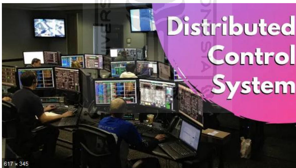
Gambar 2.2 Distributed Control System (DCS)
