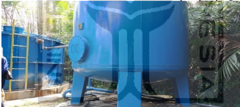
Gambar 4.1 Filter Tank IPA Kadisono
