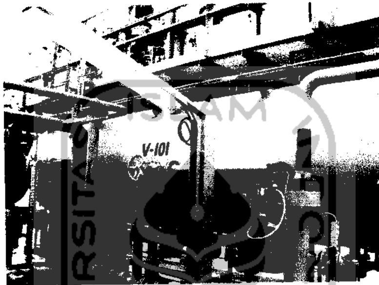
Gambar 2.3 separator V-101 ( production separator )
