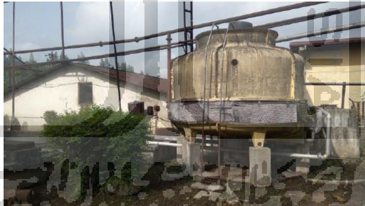
Gambar 4.13 Cooling Tray System
