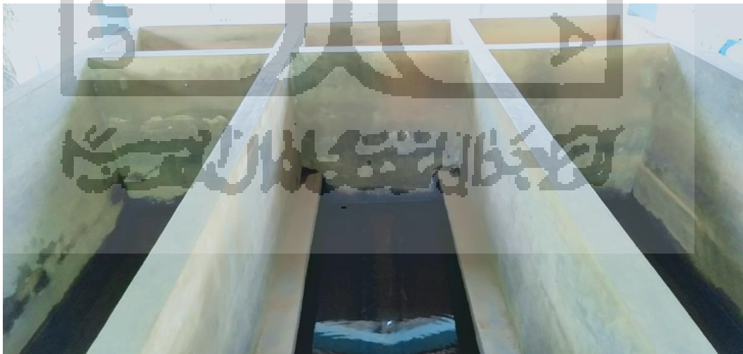
Gambar 4.42 Bak Sand Filter IPA Konvensional Cabang Depok Kregan
