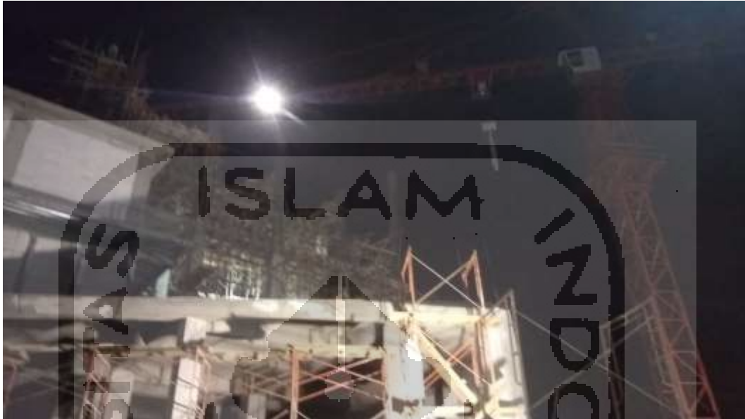
Gambar L7.1 Tower crane POTAIN FO/23B Eksisting
