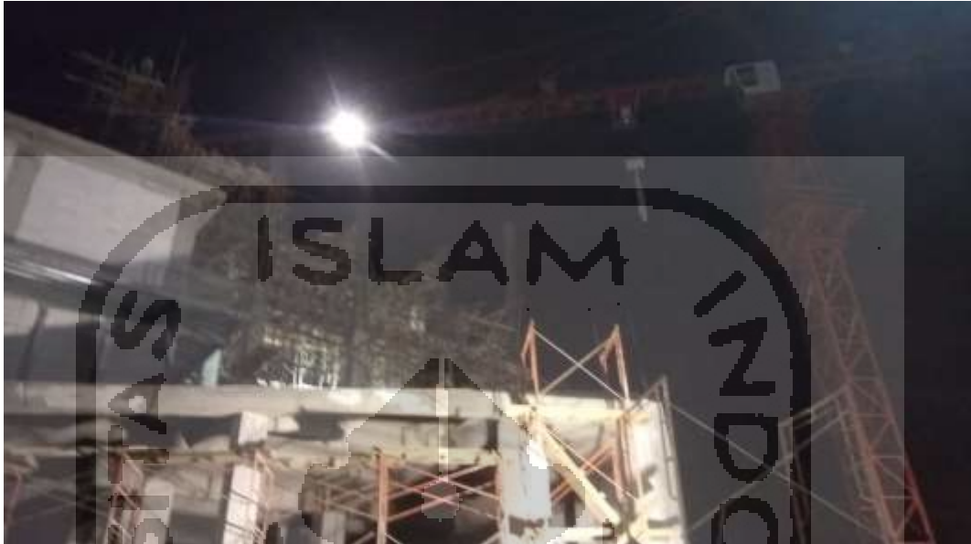
Gambar L7.1 Tower crane POTAIN FO/23B Eksisting
